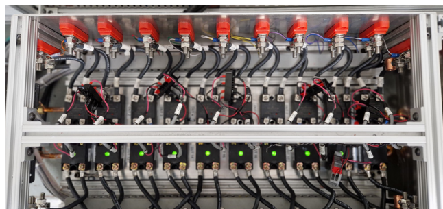
FIGURE 3. Chiller Plate with Mounted SSRs
